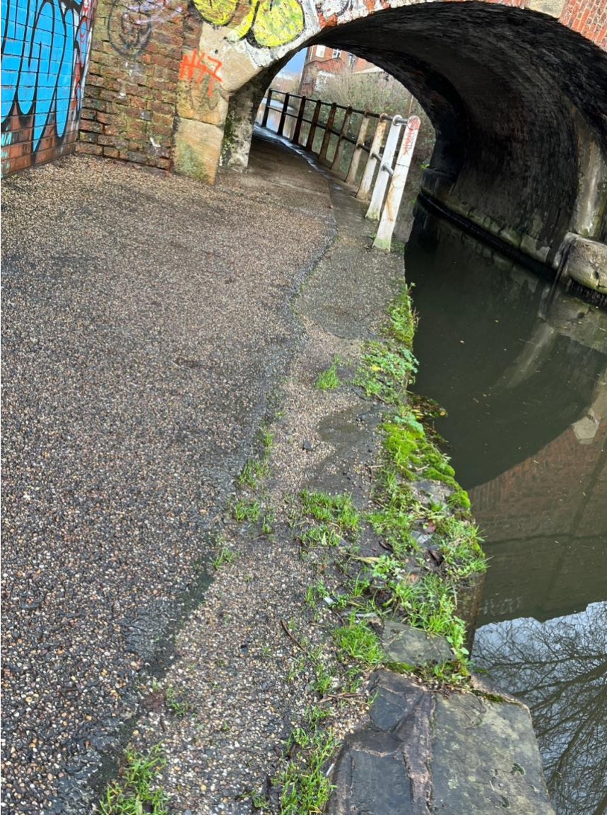
10.14 In some places, uneven surfaces from partial repairs create trip hazards next to the water.
